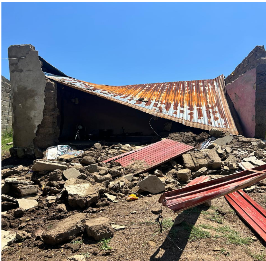
Picture: Depicts disaster damages in KwaNgedla area of Ward 13
